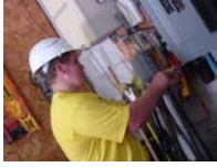
Lyle Mimbs works on an electrical panel.
